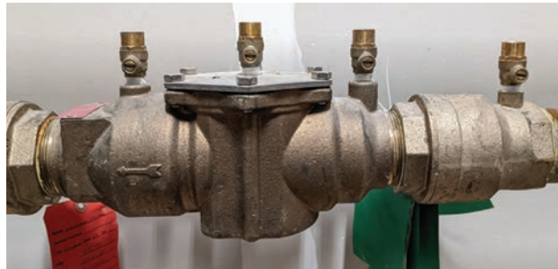
This backflow prevention device is on the fire sprinkler system at City Hall.
