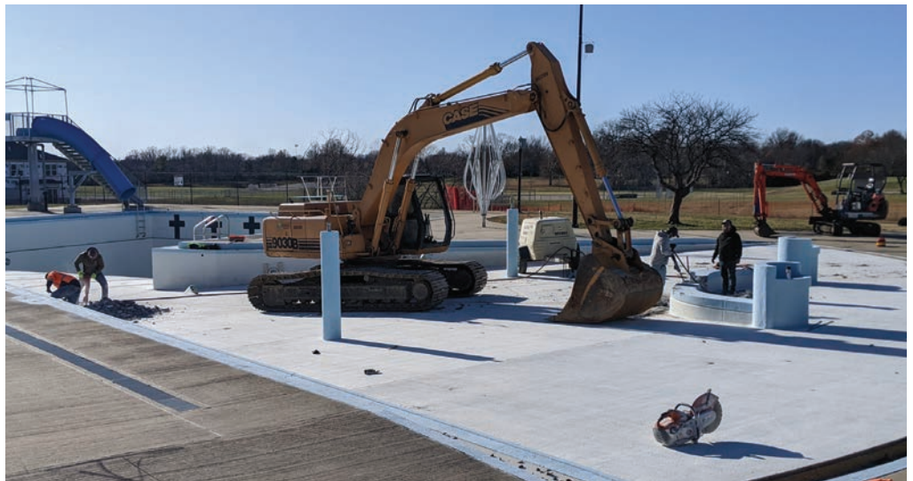
The construction company began work on renovations to the Louisburg Aquatic Center earlier this fall. The pool will see an expanded toddler play area, a rope swing for the older set, additional seating and shade areas.
