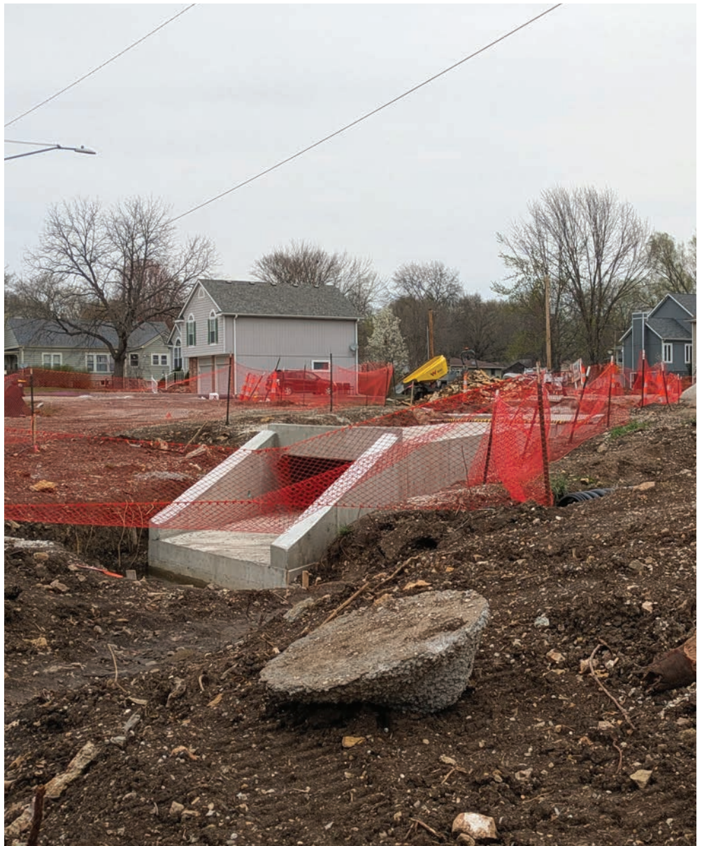
A box culvert under Rogers Road is part of a new, improved stormwater conveyance system that helps divert water from flooding streets and neighborhoods and moves it downstream. Work continues upstream to tie in all the new infrastructure.
