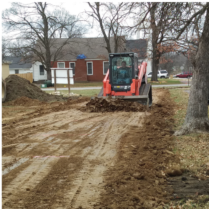
Crews work on the new sidewalk at the Farmer's Market block in late November.
