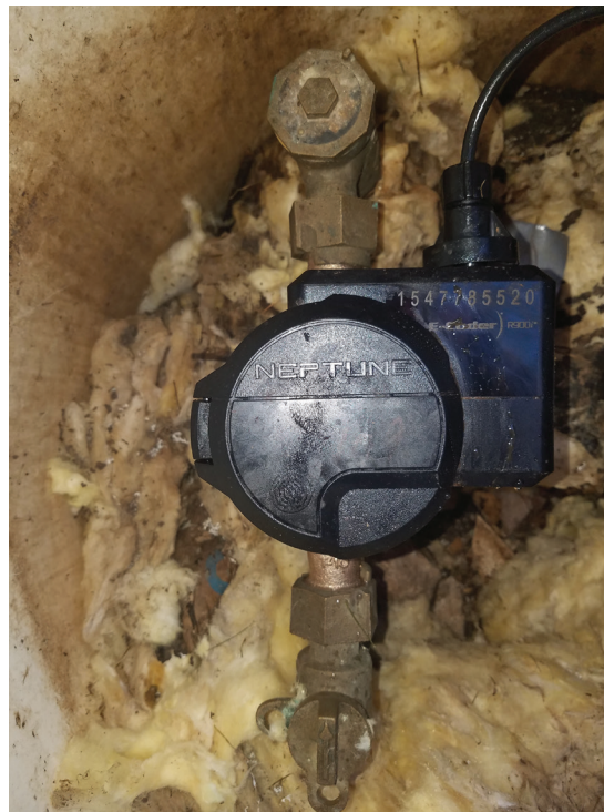
A backflow prevention device is installed in this water meter setter to prevent a contamination of the City's water supply.
