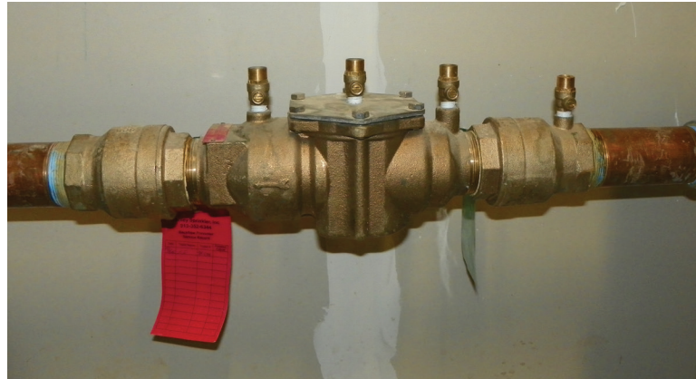
City Hall has a backflow prevention device on the fire sprinkler system in the building.
